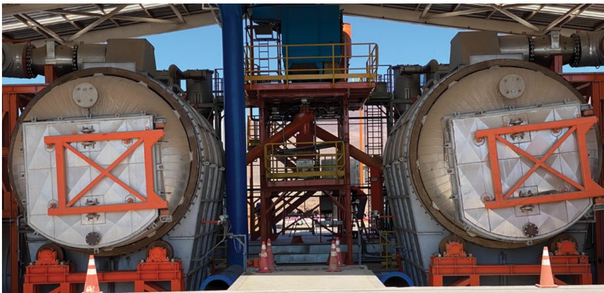
Kal Tire's thermal conversion recycling facility in Chile is the first operating facility of its kind.
